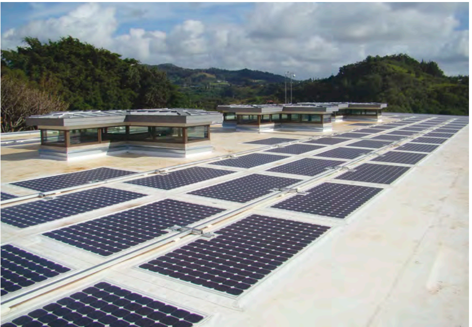
▲ An array of photovoltaic panels (PV), adjacent to clerestory windows, significantly contribute to meeting the building's energy needs. The roof also has a rainwater catchment system, allows indirect sunlight into work areas, and reflects solar heat.
